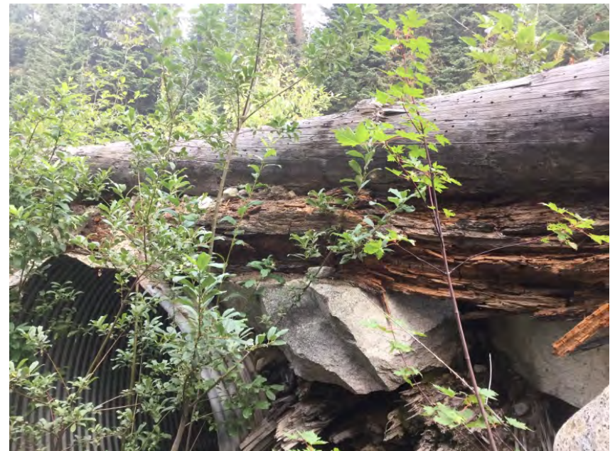
Rotten fender logs
