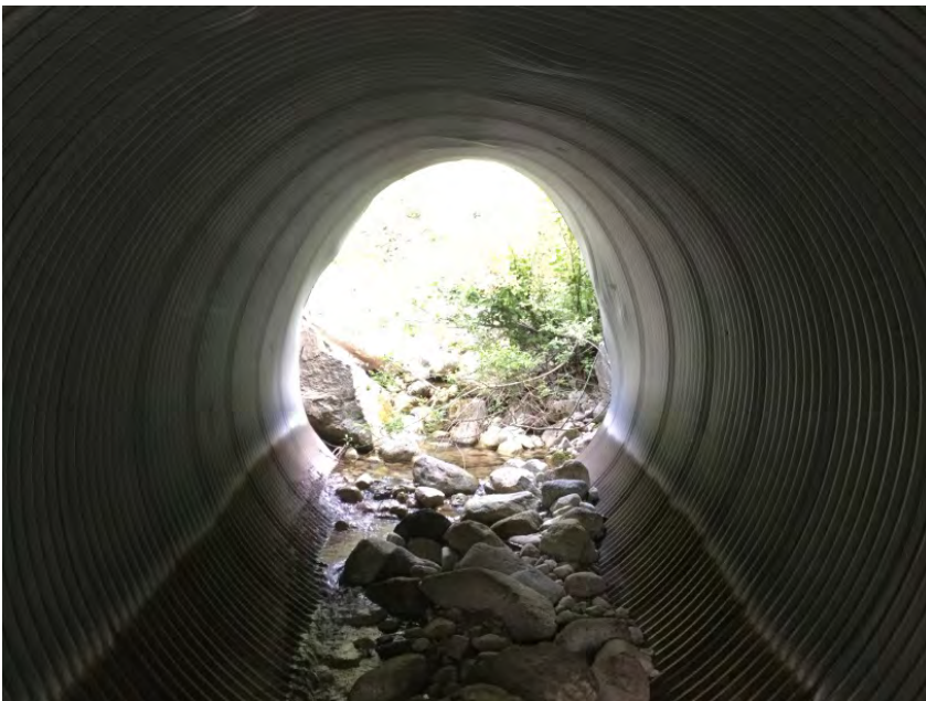
Deformation at inlet
